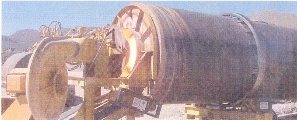
Asphalt Kiln with Ferox (Ferox improved fuel efficiency 14%)
